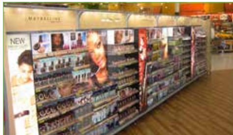
LED rail cornice lighting
